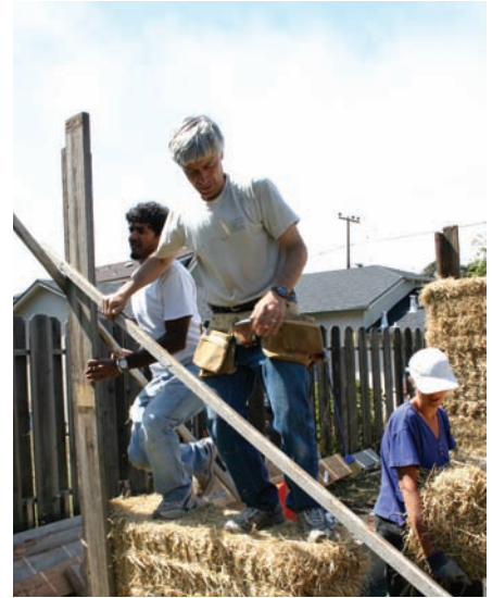
VOLUNTEERS PUT ONE OF THE FIRST BALES IN PLACE IN THE SMALL STRAW BALE YOGA ROOM, PACIFICA. Courtesy of San Mateo County Recycle Works
